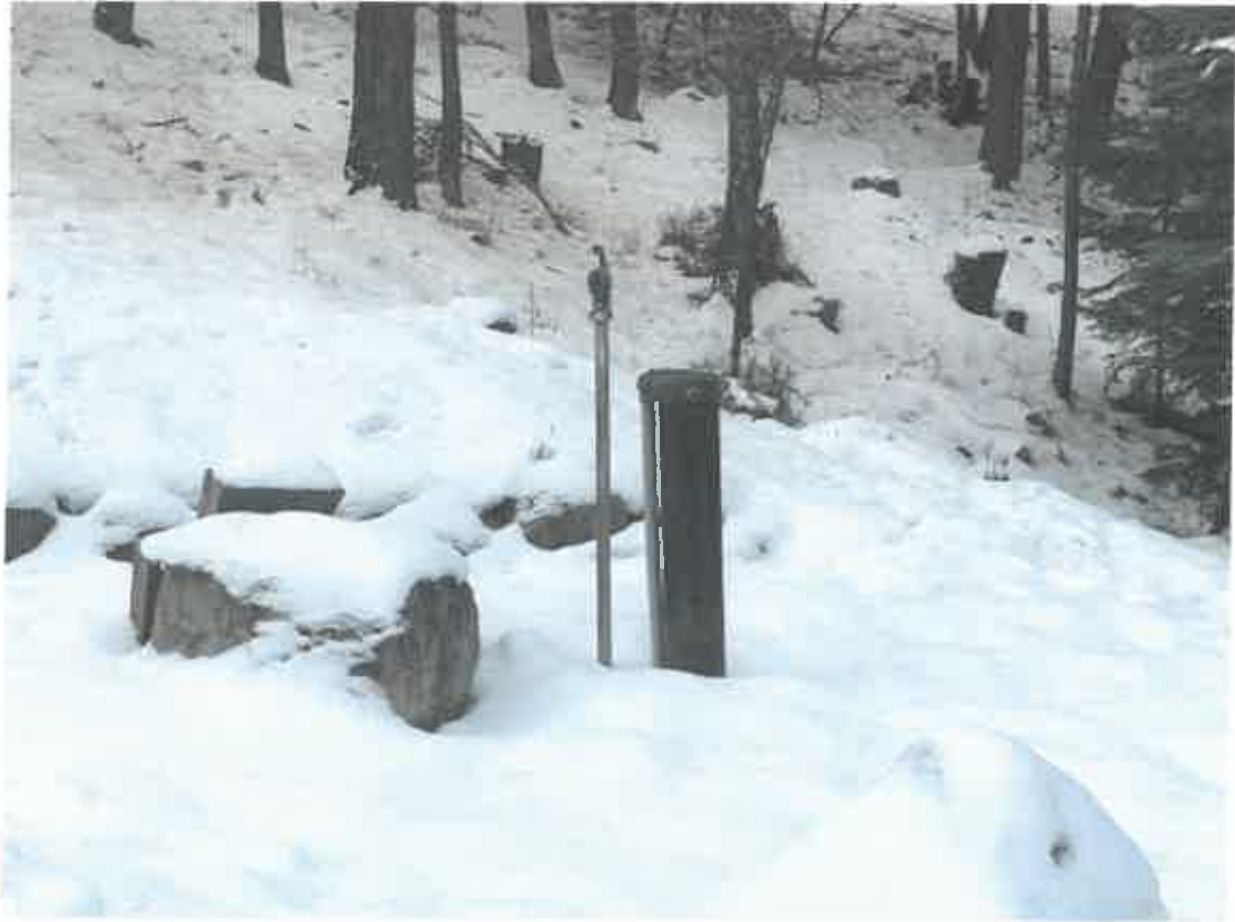
Ground Water Well at 130 Spotted Fawn Lane
