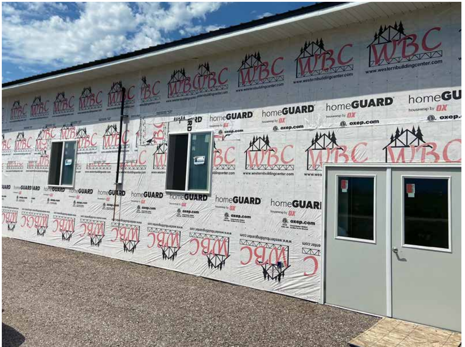
The construction is near completion on H and D Meat Processing's new facility funded in part with the Department of Agriculture's Montana Meat Processing Infrastructure Grant program. Photo by Marty Earnheart
